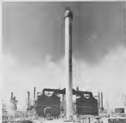
New furnace stack of Pipestill 5 and 6 nearing completion. Schoorsteen nobo pa fornu di Pipestill 5 y 6 binlendo cla.
